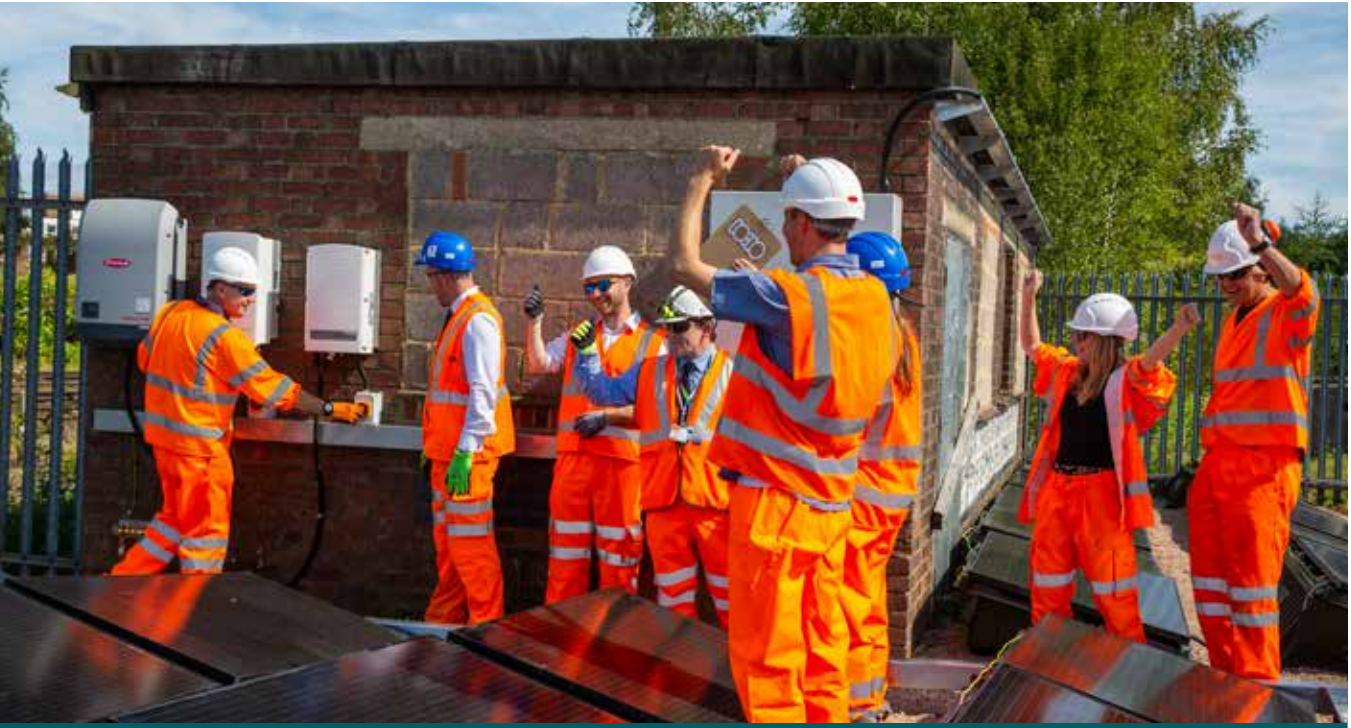
Basingstoke companies were in a world first in 2019 as solar power was connected to railway lines. Basingstoke Energy Co-operative, working alongside Network Rail engineers, took a leading role in the design and implementation of the system known as Riding Sunbeams. Credit © Andy Aitchison / Riding Sunbeams
